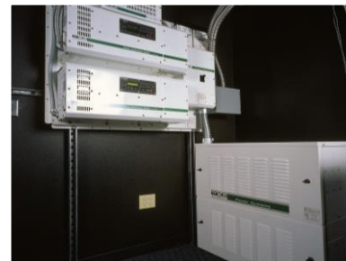
Battery energy management systems
